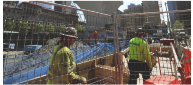
The Rainier Square development is under construction in downtown Seattle. (Alan Berner / The Seattle Times)
